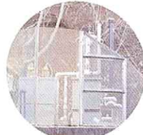
Drain water -recycling system. (Drainage Tank is buried underground.)
