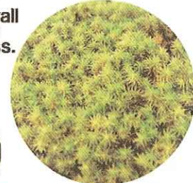
Roof and wall covered by moss.
